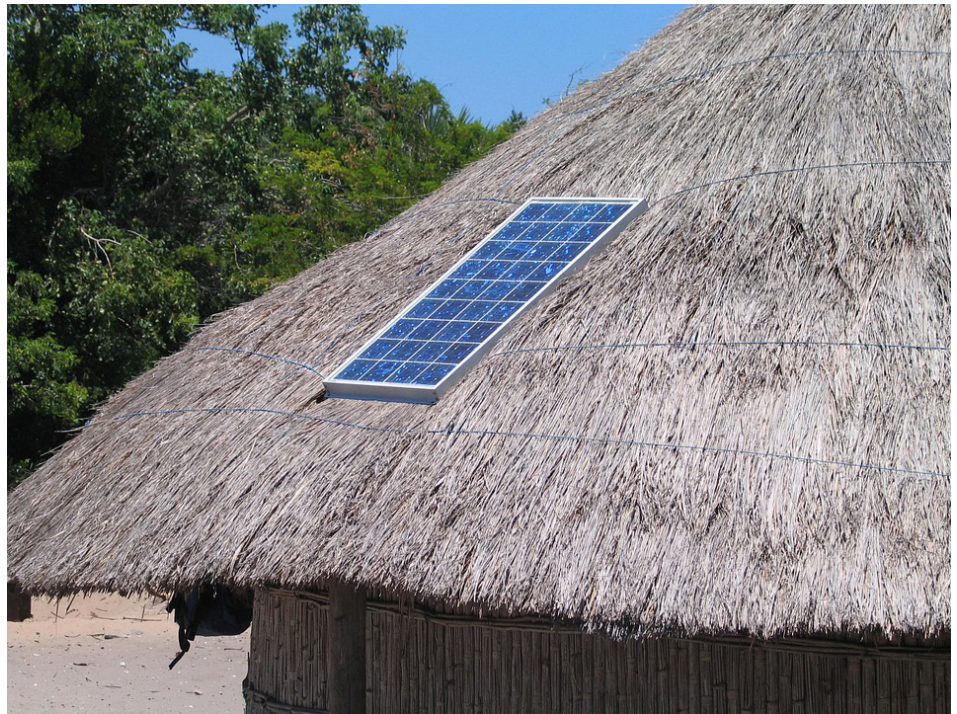
Solar Panel on Straw Hut Roof by Teresa Cotrim (cotrim), 2005, used under Pixabay license, accessed 16 July 2019.
